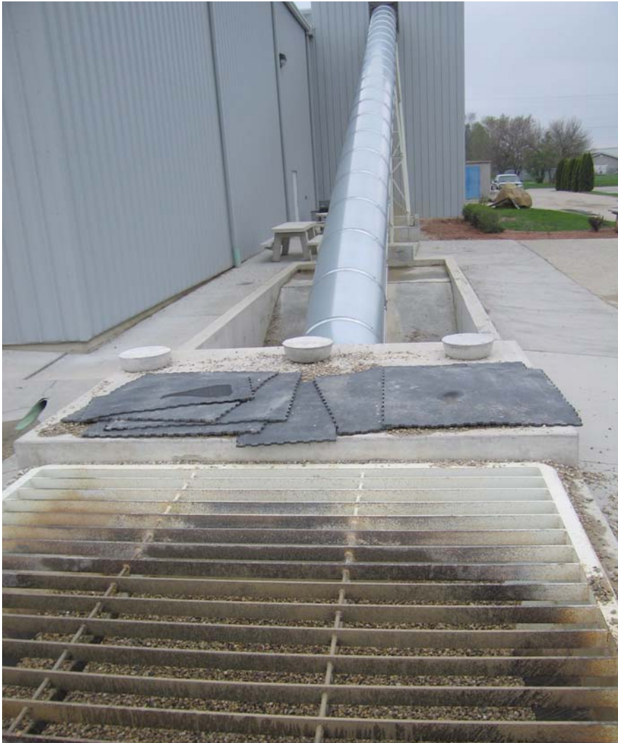
Below grade aggregate grizzly enables efficient charging of the 2-compartment indoor aggregate silo directly from a truck or frontend loader – no double handling required.
